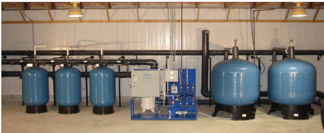
Figure 6.2. Chemical water treatment system
