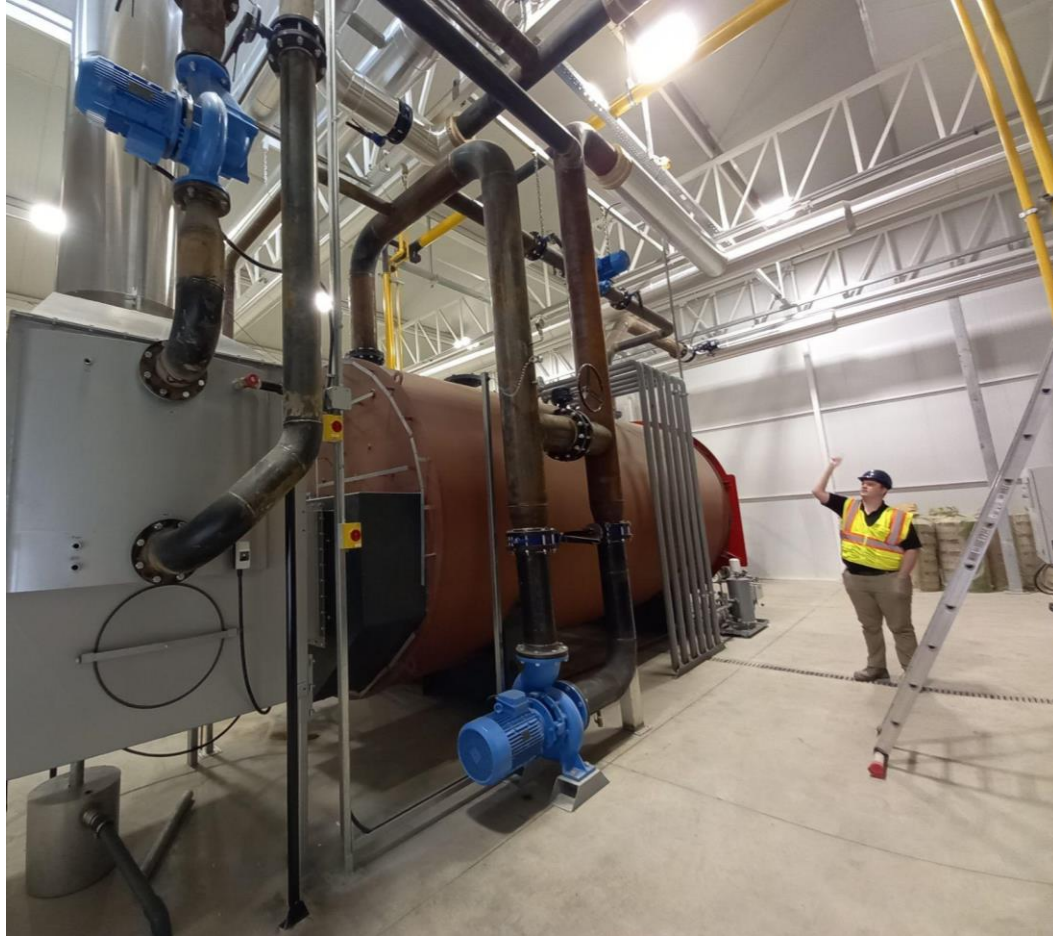
Figure 8.5. Boiler system in the mechanical room of a greenhouse facility
