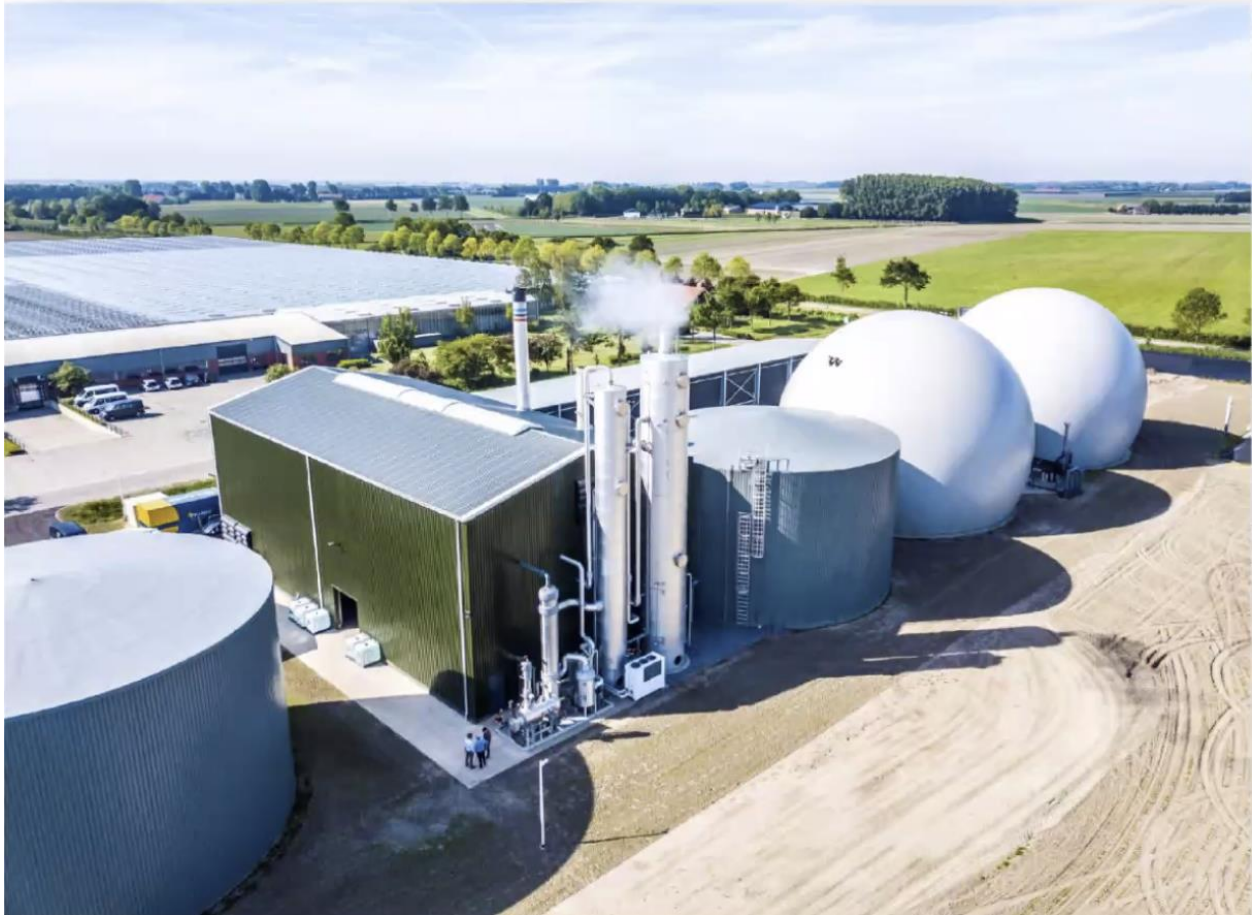
Figure 10.6. CHP exhaust capture and cleanup system for use inside the greenhouse
