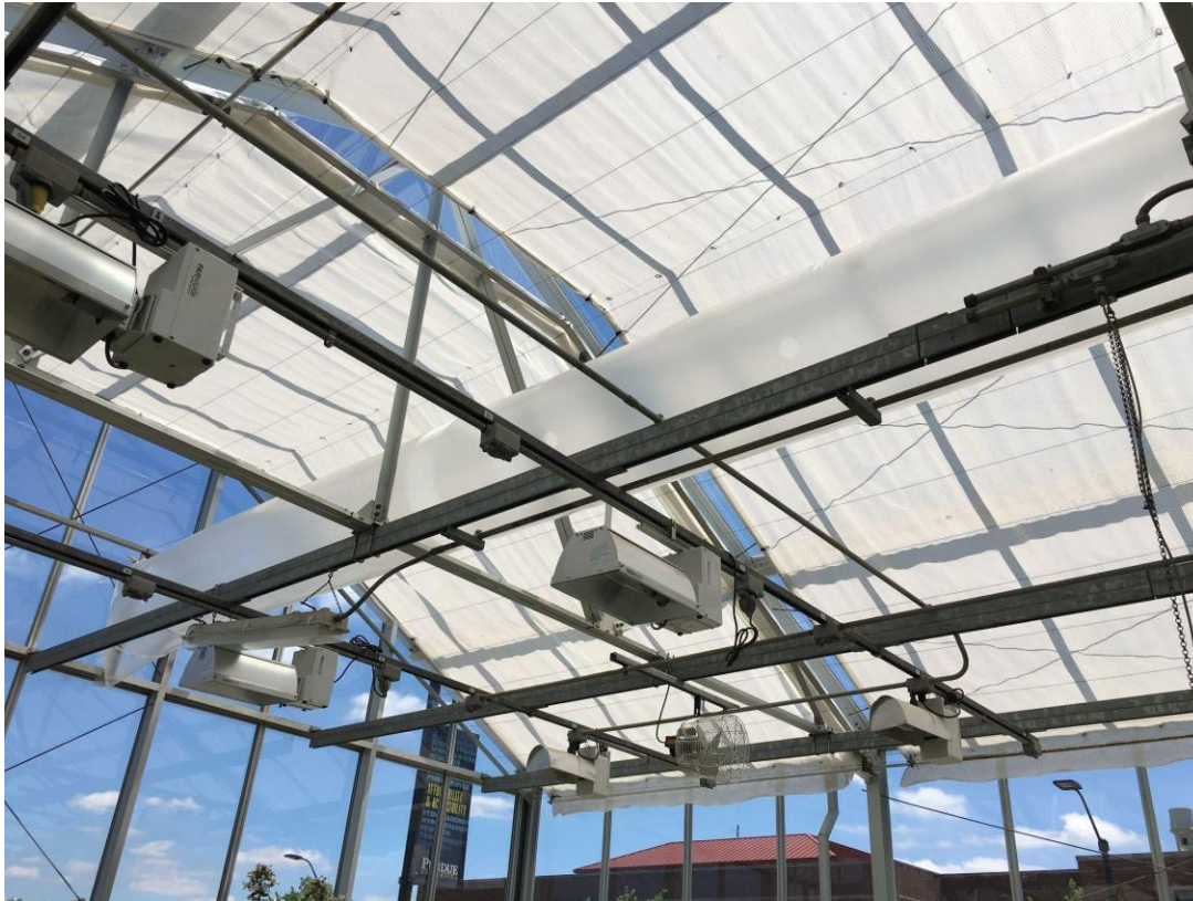
Figure 8.4. Greenhouse ventilation view from inside
